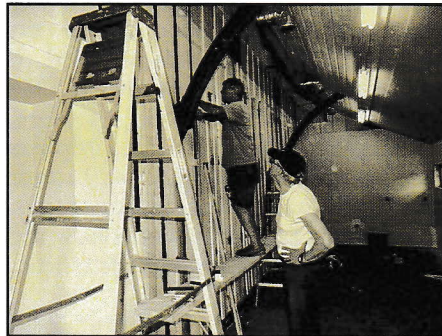
Bernie Hanmore and Ed Cronin installing drywall in the kitchenette at the Meadville Railroad Depot. (Jack Sheets photo)
