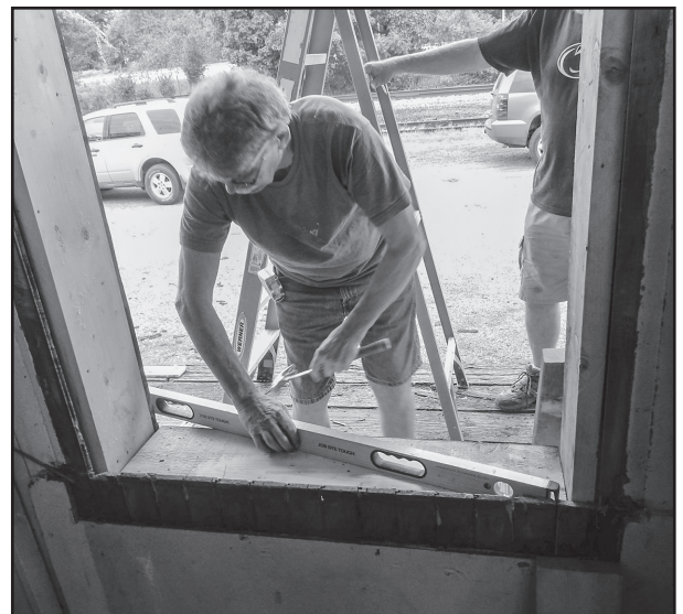
Bernie Hanmore prepping the sill of a new window at the depot. (Maryann Martin photo)
