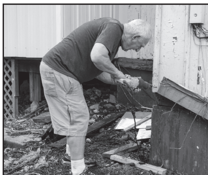
Arden Hibbard working to stabilize an extended section of the depot. (Maryann Martin photo)
