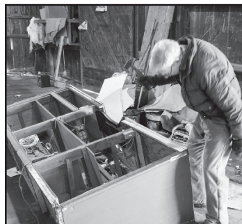
Ed Cronin breaking apart a counter that once served the Meadville Farm & Garden. The counters and shelves are being cleared out to make room to renovate the former B&LE freight and passenger depot into a museum. - photo Nick Ozorak
