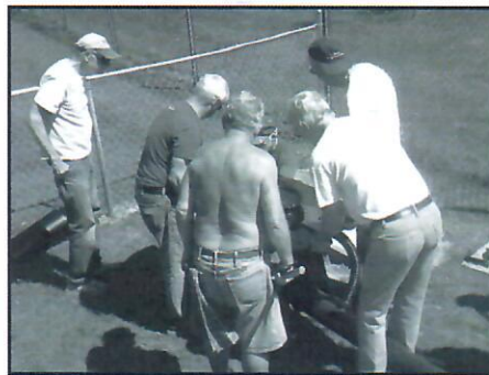
Work crew attaching the signal head to the pole - August 8, 2017 (Photo by Carl Timko)
