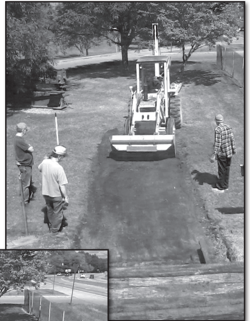
Terry Martin grading and removing the sod in front of the 518 with his front loader.
