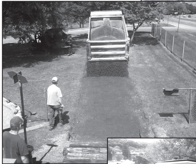
Kebert's Construction dumping a load of 2RC gravel for a base for the track panel to rest on.
