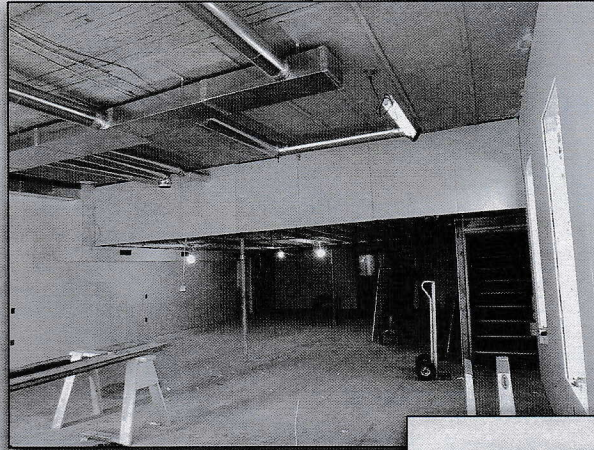
Interior of Depot after drywall has been hung. (Photo by Maryann Martin)
