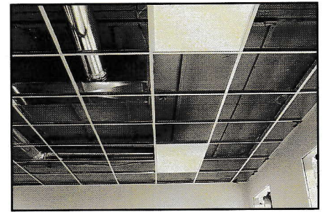
Grid work of lowered ceiling with LED light panels installed. Main room November 10, 2020 - ©FCVRRHS
